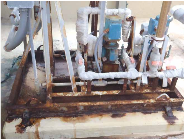
Example of a rusting acid skid
